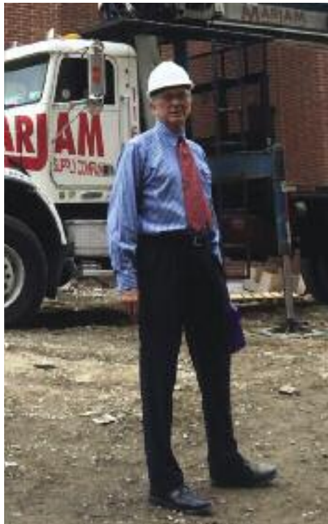
Feuerstein on the Barrier Free Living construction site in the South Bronx.
